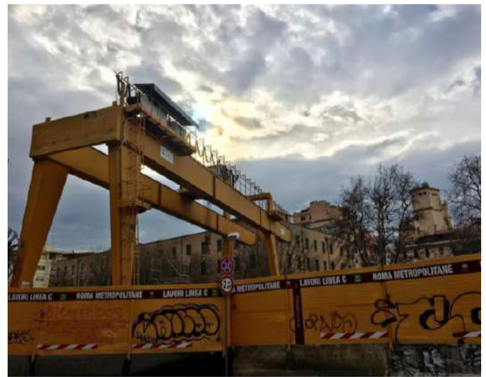
The construction has created many issues with maintenance in the neighborhood
