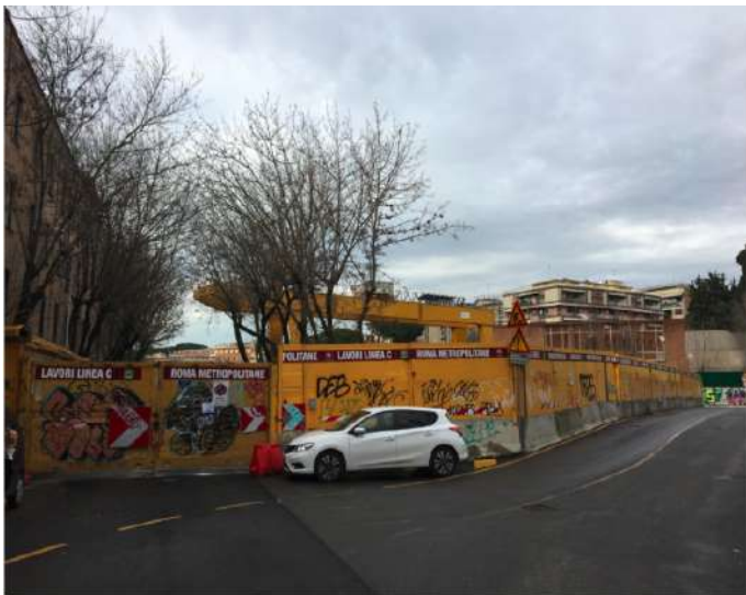
Image of the construction currently taking place in San Giovanni for the Metro C
