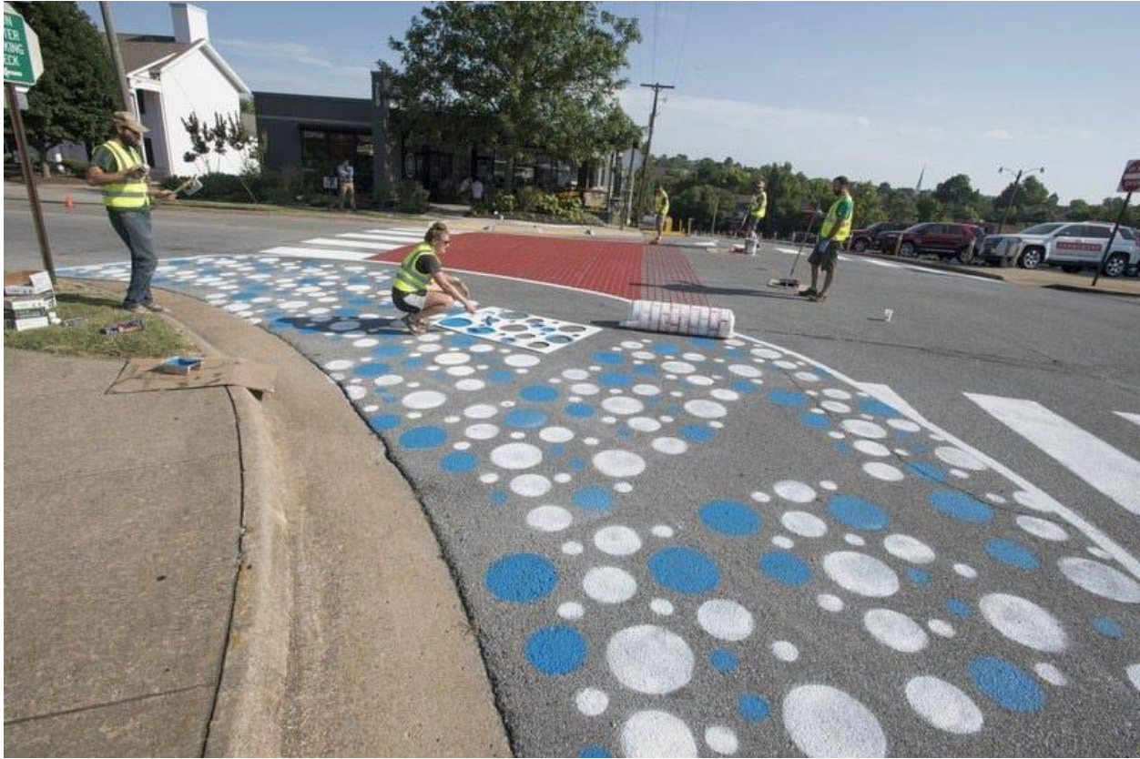
Figure 5: Volunteers in high-visibility vests paint a polka dot pattern around a curb and two-way crosswalk in Fayetteville, Arkansas. Source: Fayetteville Department of City Planning.
