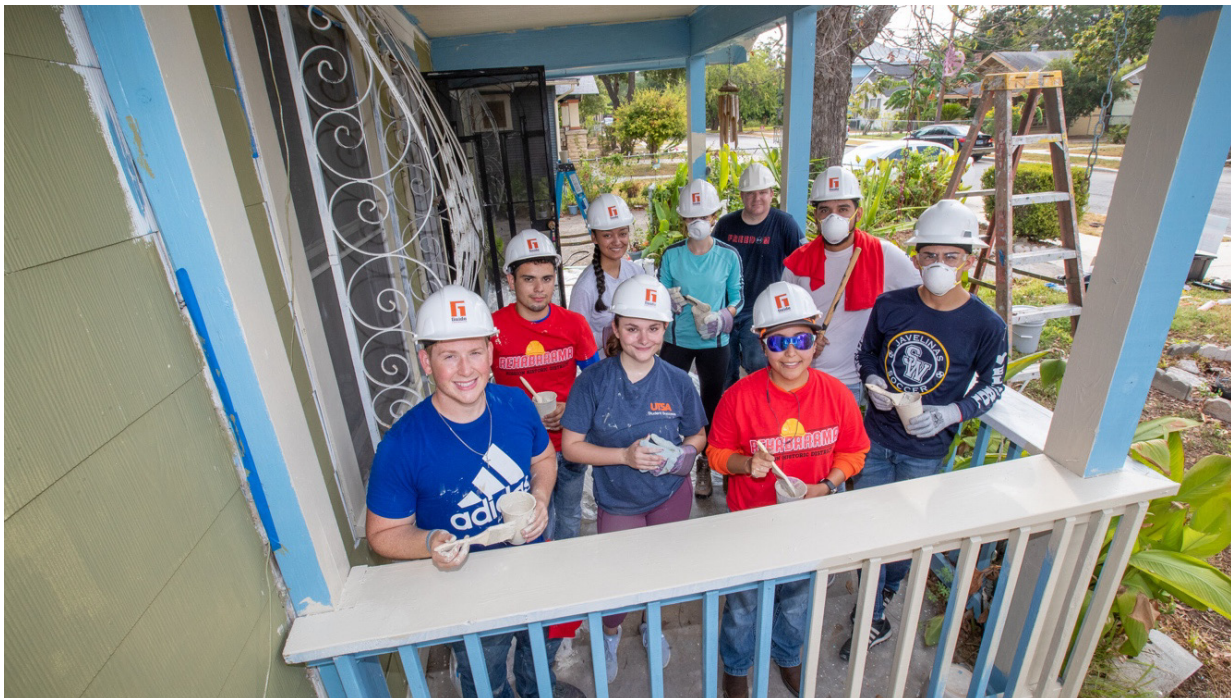
Image 1. Twice a year in San Antonio, the Rehabarama program brings together neighborhood residents, volunteers and local contractors to repair aging homes. Launched by the city's Office of Historic Preservation, it allows people to remain in their homes longer while creating generational wealth. Frederick Gonzales, courtesy of City of San Antonio.
